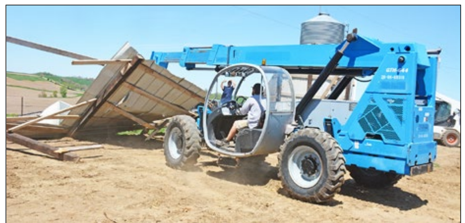
This piece of equipment was used to pull down the walls of a demolished shed at the Denise Christensen place.
